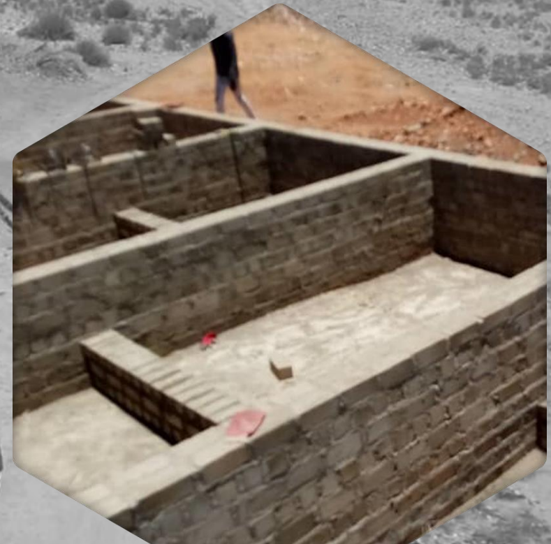
Water Filtration System
